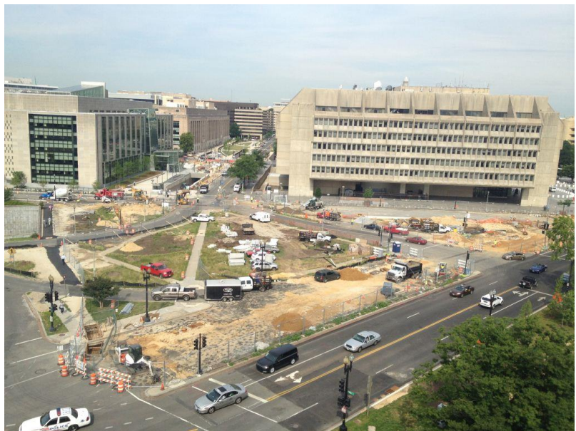
Construction is under way at the site of The American Veterans Disabled for Life Memorial in Washington, D.C. Anticipated dedication date is October 12, 2014.
